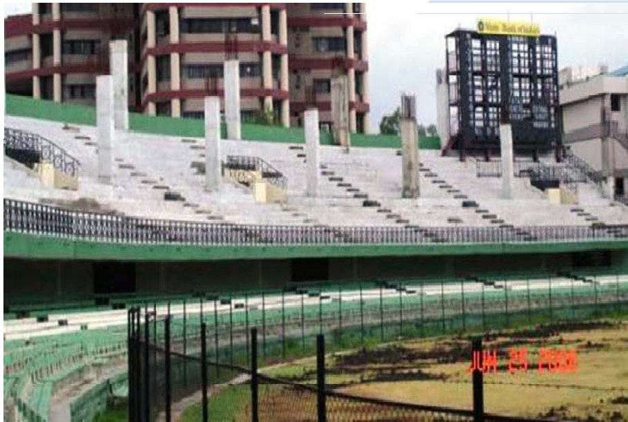
Tier 1 and 2 of stands in place with columns for tier 3 coming up
